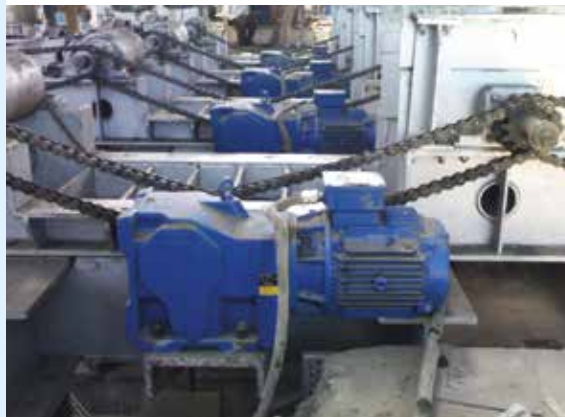
Bevel geared motors for cooling bed chain feed tables
