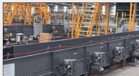
BCS solution for Toll IPEC facility Melbourne
