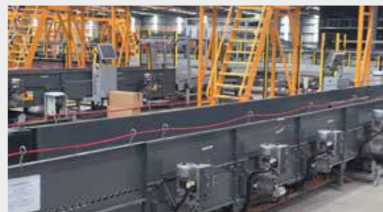
BCS solution for Toll IPEC facility Melbourne
