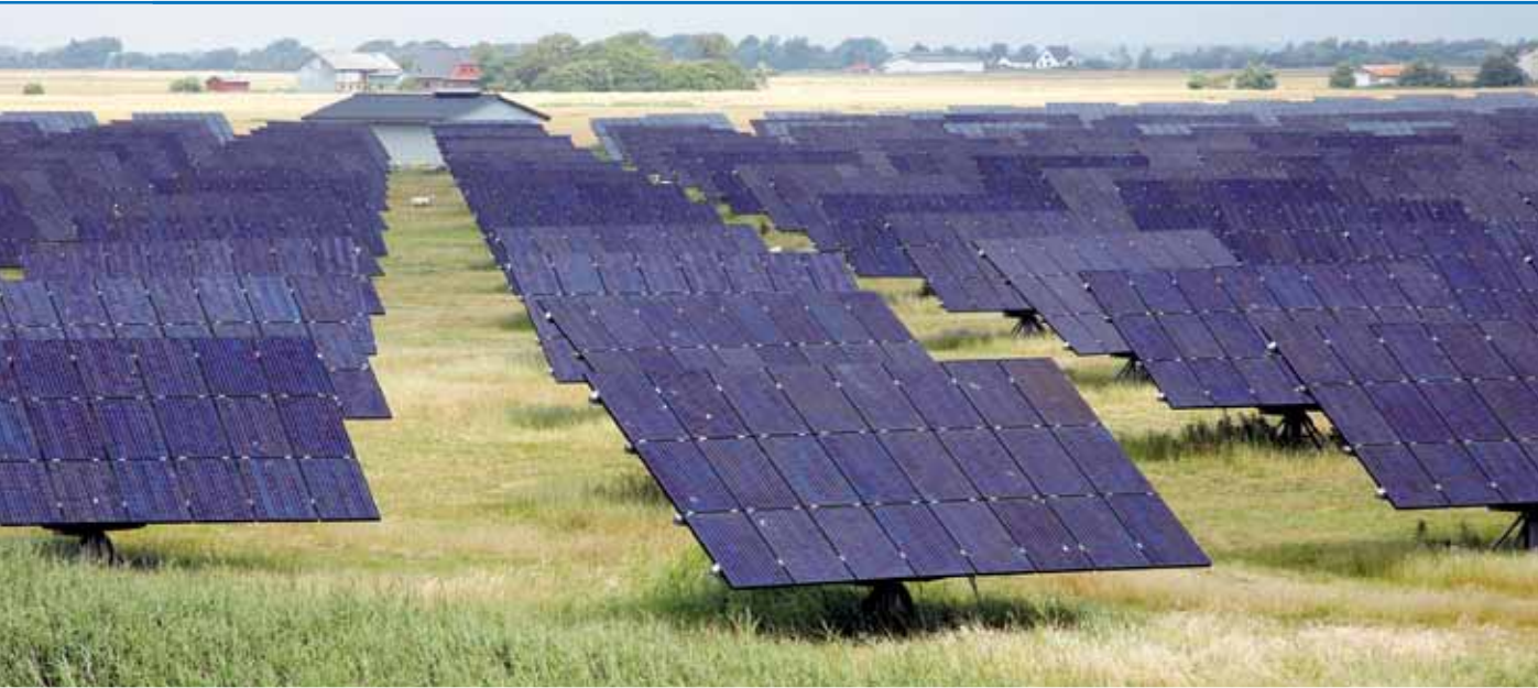
Green technology in the far north of Germany: Rodenäs Solar Park, with more than 700 solar modules.
