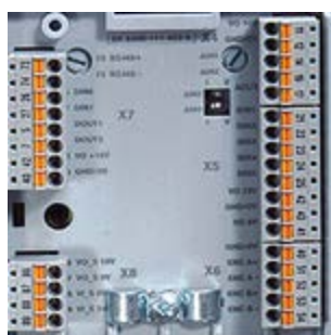
Figure 4: EMC kits installed for control cables
